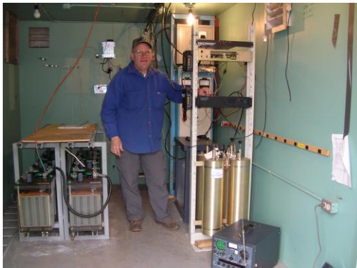
Gary (VE7LCP) proudly showing newly installed 146.88 repeater, duplexer, charger (above his right shoulder) and link radios (mounted sideways on outside of rack).
